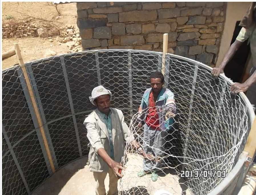
Picture 15: Lining of the wire mesh along the inside of the body mold.
